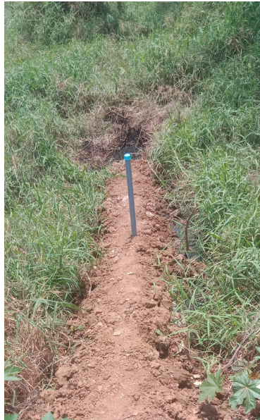
Fig 14: Pipe markers along pipeline
