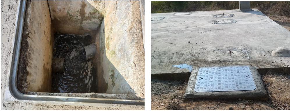
Fig 7: Inlet unclogged (left) and FRP sheet top lid for the inlet (right)
