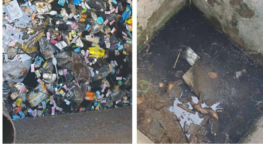
Fig 9: Manholes filled with plastic and sludge
