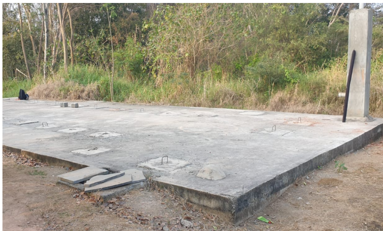
Fig 6: Broken inlet before intervention
