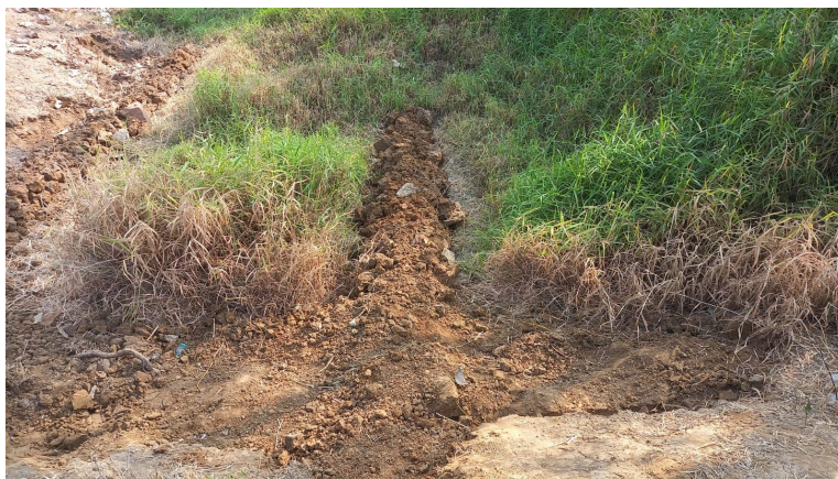
Fig 10: Pipeline supported and covered with soil
